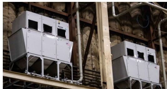
BIW's new high-efficiency air filtration units.
