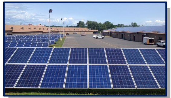
Financed through the CT Green Bank with assistance from RGGI funds, the solar PV system at Sofia's Plaza is expected to save $153,183 in annual energy costs. Photo Credit: Connecticut Green Bank
